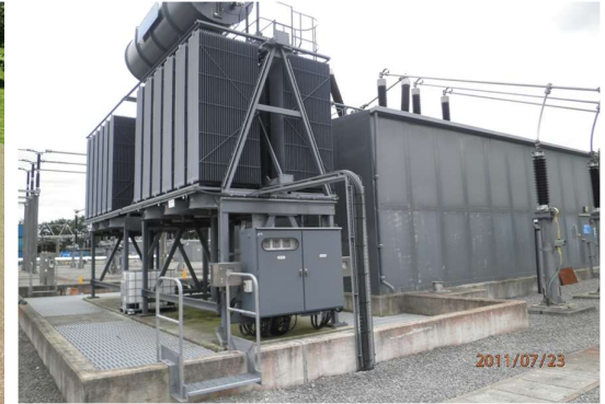
400 kV Power Transformer
