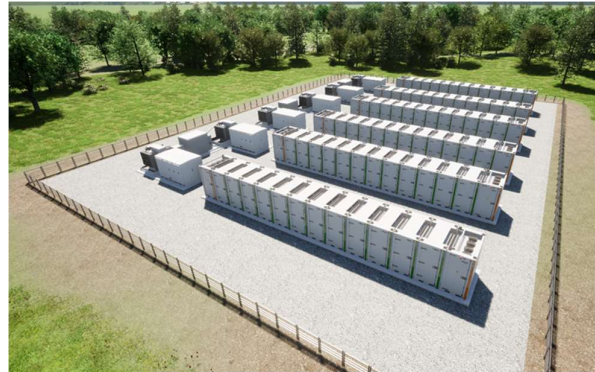
Battery Storage Compound
